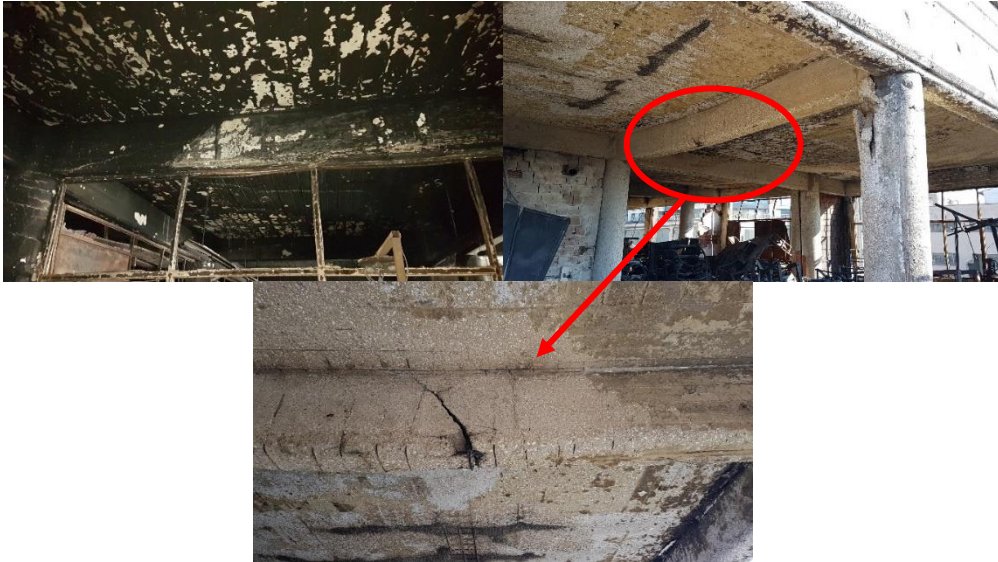
Fig. 17 Deformed beams at Ground and 1 st floors
