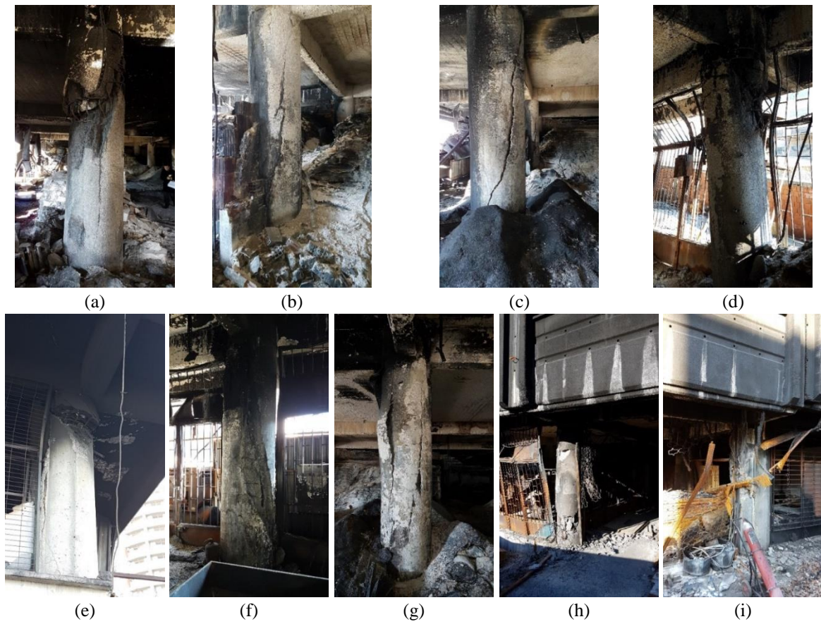
Fig. 9 Failures of the several columns at the 2 nd basement
