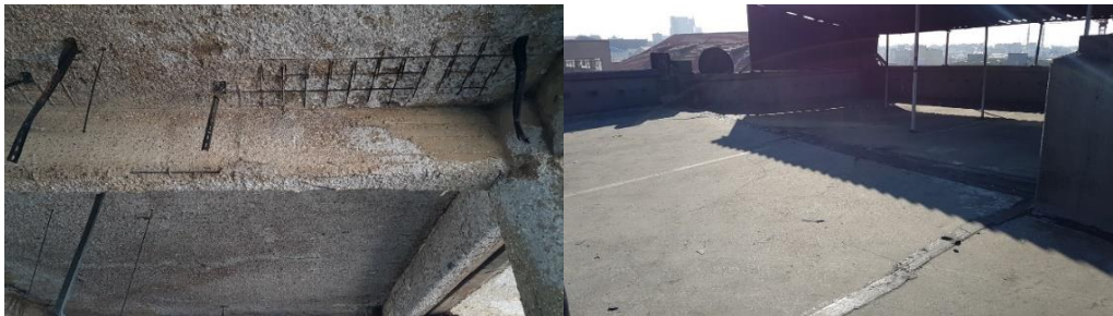
Fig. 20 Spalling and bared reinforcement at 1 st floor and deep cracks on 2 nd floor slabs
