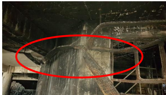
Fig. 13 Shear wall beam cracks on 2 nd basement
