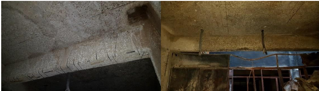
Fig. 16 Spalling of beams and visible reinforcements on the ground floor
