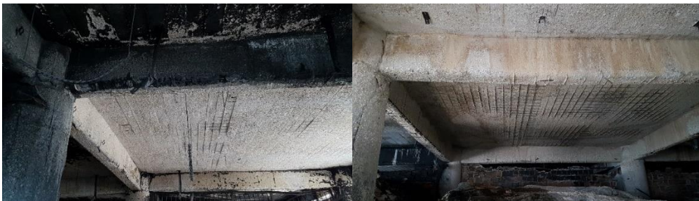
Fig. 18 Spalling of slabs and visible reinforcements at the 2 nd basement
