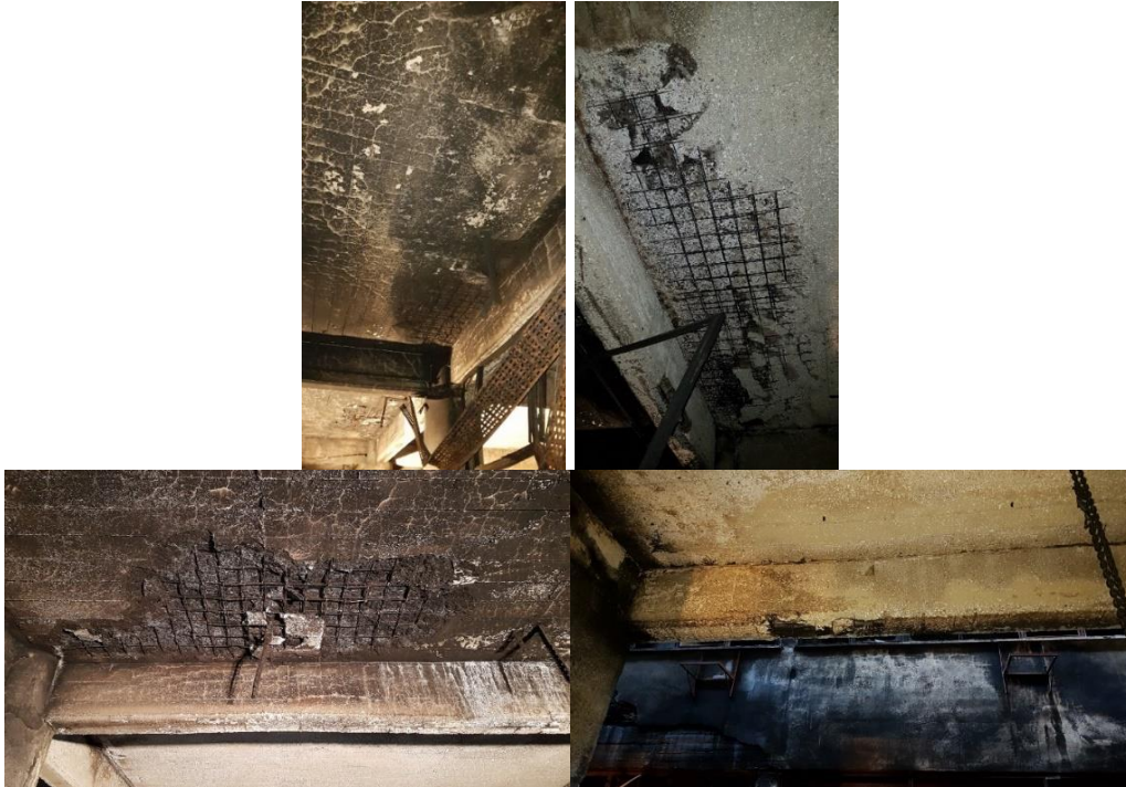
Fig. 19 Net-like cracks, spalling and bared reinforcements at 1 st basement slabs
