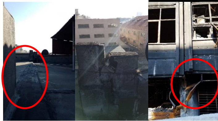
Fig. 11 The displacement of Block 5 relative to Block 4 from the roof of the building
