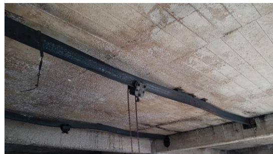
Fig. 23 A deformed steel roof rail at 1 st floor
