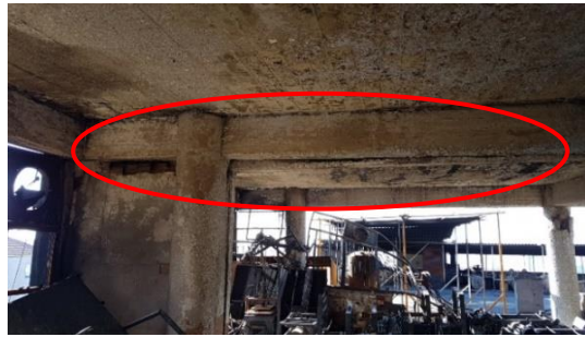
Fig. 12 The displacement of Block 5 relative to Block 4 from inside of the building (shot on 1 st floor)
