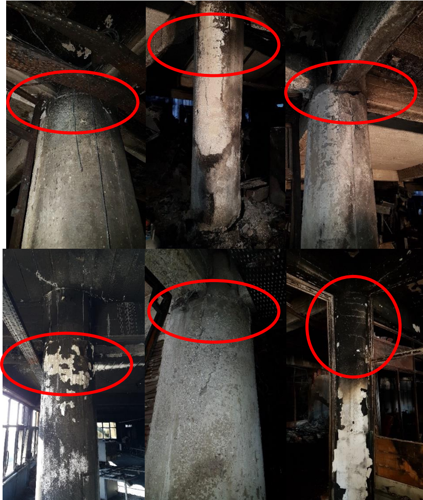
Fig. 14 Connection cracks on the 1 st basement and ground floor
