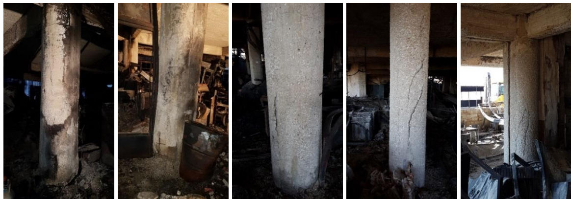
Fig. 10 Cracks of several columns and spalling on the 1 st basement and 1 st floor
