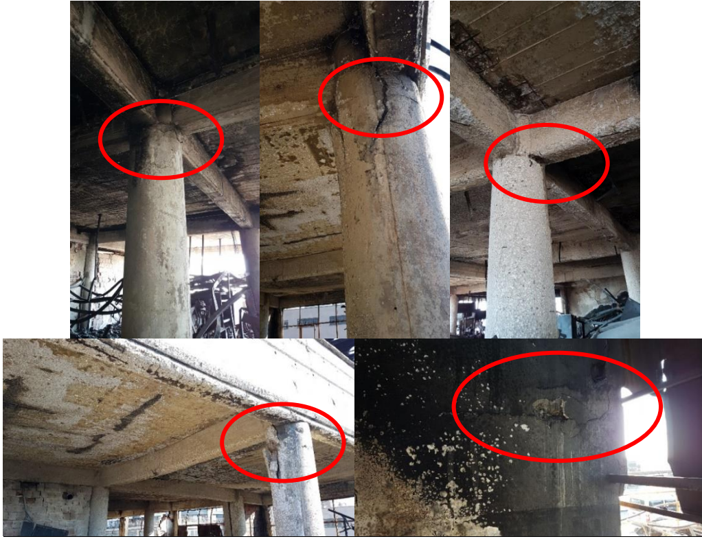
Fig. 15 Connection cracks on the 1 st and 2 nd floors
