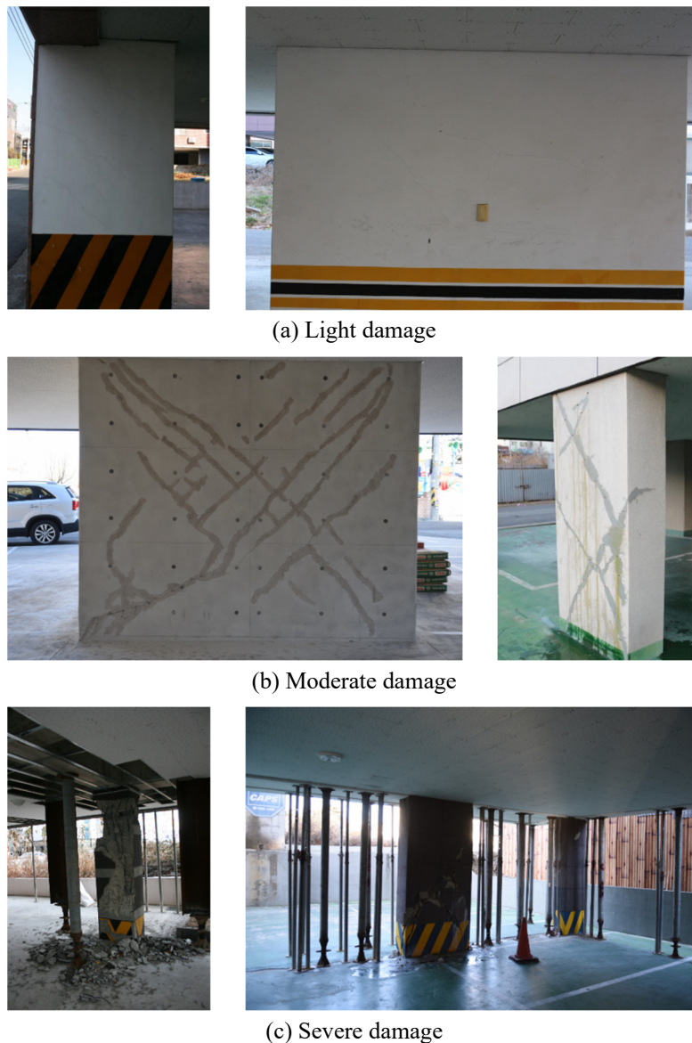
Fig. 10 Pictures of damaged buildings (Sim et al. 2018)
