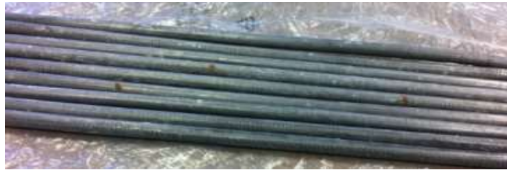
(a) Bare steel bars of a beam
