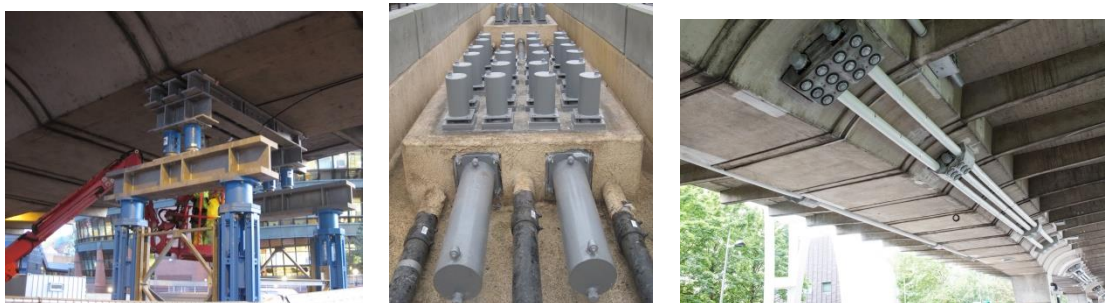
Fig. 11 Temporary propping during investigations (left), new external post-tensioning across critical spans (middle) and additional strengthening (right)
