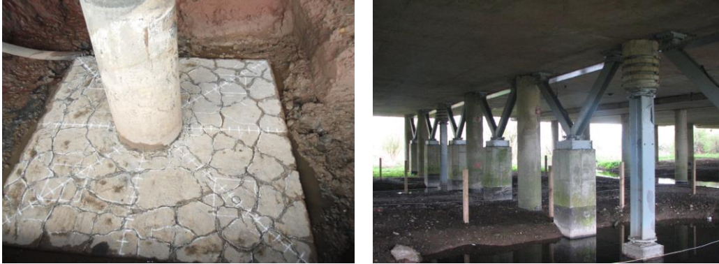
Fig. 13 Alkali-silica reaction on a footing of a pier of Floodplain #2 (left) and piers subjected to full scale tests on the grid-line S (right). (Courtesy: Highways England)
