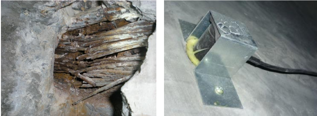
Fig. 8 Failed wire strands (left) and acoustic emission sensor (right)
