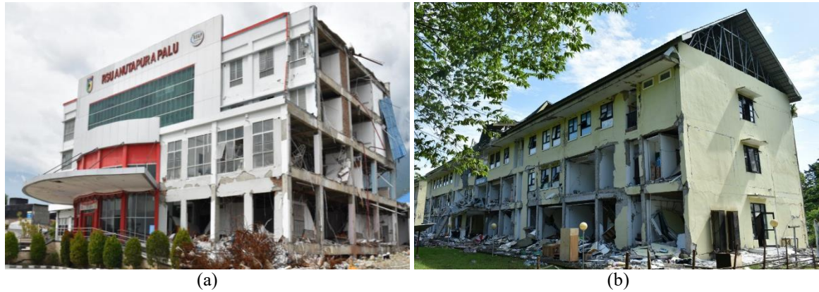
Fig. 1 Post-earthquake damages (a) Hospital building in Palu Earthquake 2018 and (b) Residential building in Mamuju Earthquake 2021
