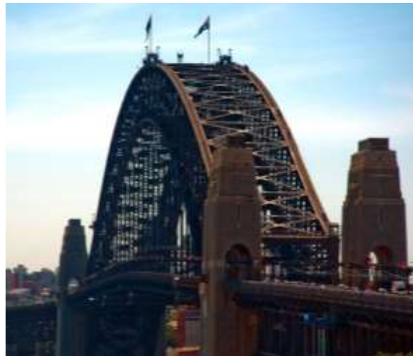
Fig. 2 Data capturing - Location 1: on the top of the lower arch and Location 2: near the bottom of the north pylon (Australia 2010)
