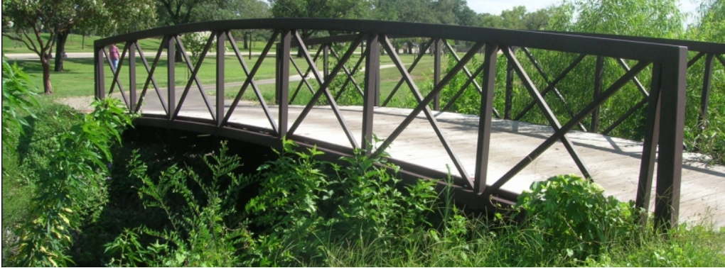
Fig. 6 Pedestrian bridge in Texas A&M Golf Course at Texas A&M University, College Station, TX
