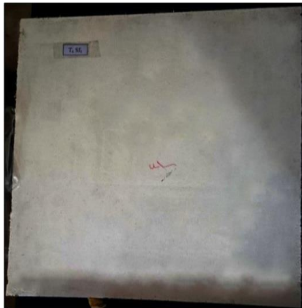
Fig. 4 Crack pattern of the slab T4SF1
