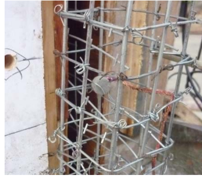
(b) The sensor embedded in the column
