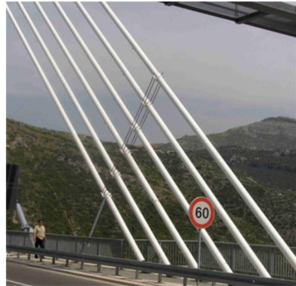
Fig. 10 Adaptive cable damper (ACD) installed after the May 2006 snowstorm (2 ACD-140 clusters each for 6 back stays)
