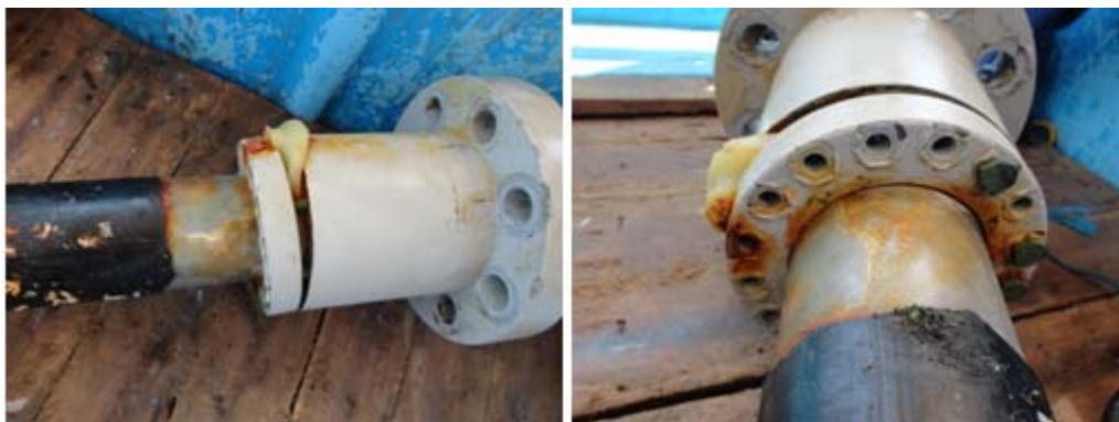
Fig. 4 Damaged smart flanged removed from the sealine
