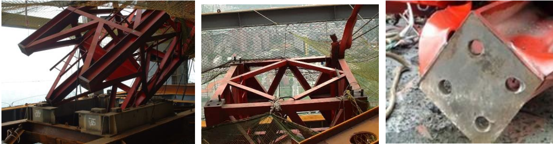
Fig. 2 Destruction of a tower crane mast of a high-rise in Taiwan
