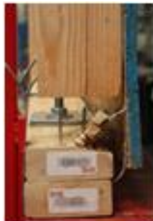
(a) Torn out OSB, withdrawn nails and combination of several failure modes
