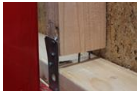
(b) Failed frame connection and LSTA 9 tie fastener nail withdrawn
