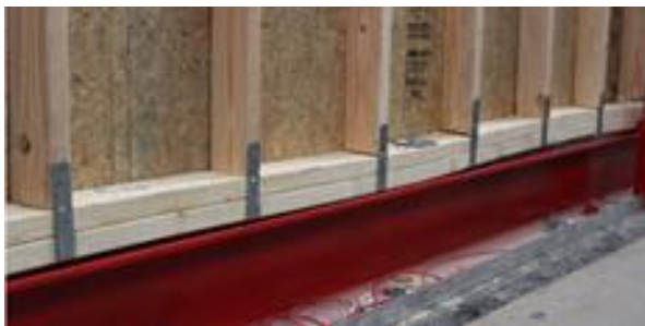
(a) Bent baseplates
