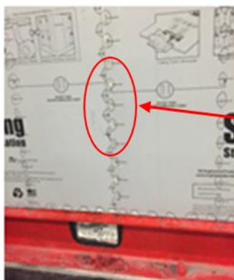
(a) Failure of structural foam panel due to bearing of staples through the pane
