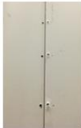
(b) Failure of GWB due to bearing of screws through the GWB
