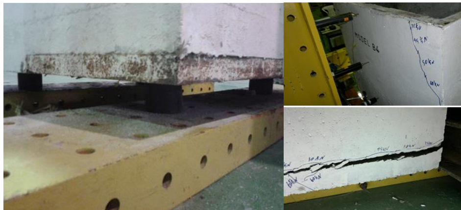
Fig. 11 Damaged state of the FB and HDR specimens at the final step of the pushover test
