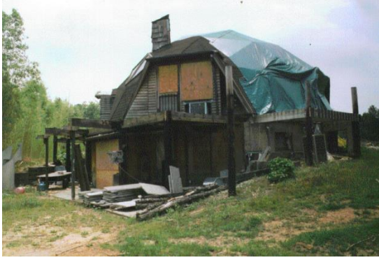
Fig. 2 Dome survived with partial failure (New Age Dome Construction , 2016)
