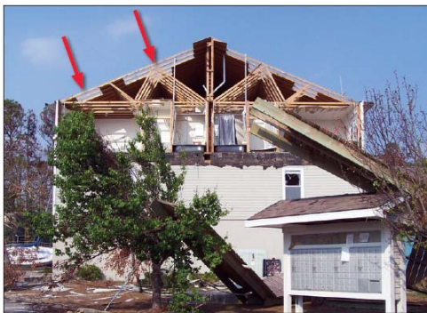
(c) Gable end wall and roof edge sheathing (arrows) failure in Katrina (FEMA 2006)
