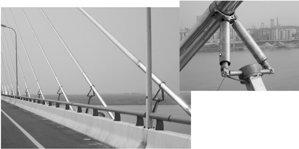
Fig. 3 MR damper installation on the Dongting Lake Bridge, Hunan, China
