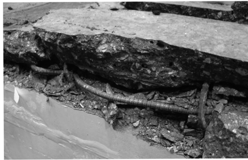
(a) Crushing of concrete, buckling of compressive steel, and slip of hook in stirrup
