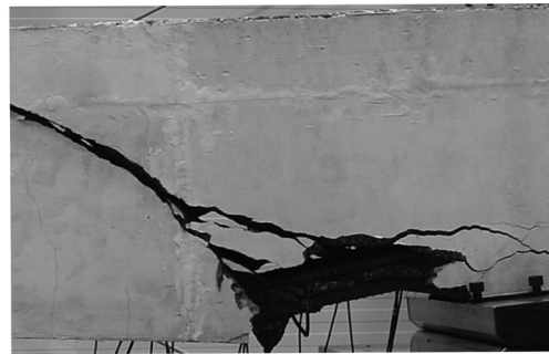
(b) Shear-splitting crack
