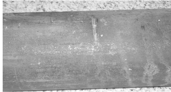
Fig. 10 Damage situation in No.7 element of No.2 pipeline
