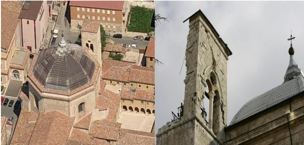
Fig. 3 San Bernardino church in original conditions and observed damage after the 6.3 magnitude earthquake of L'Aquila, Italy on April 6th 2009
