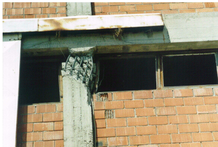
Fig. 10 Short column effect in the case-study building
