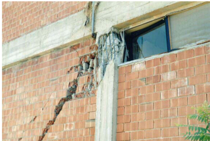
Fig. 2 Another example of short column failure in 1998 Adana-Ceyhan earthquake in Turkey
