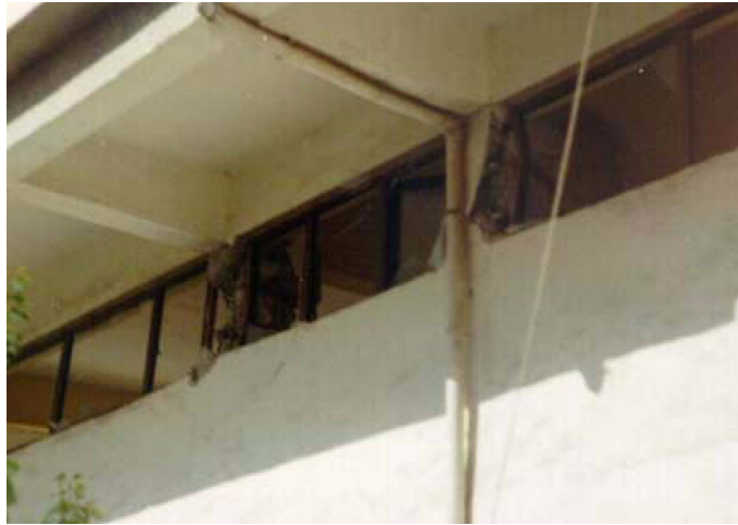
Fig. 1 An example of short column failure in 1999 Kocaeli earthquake in Turkey
