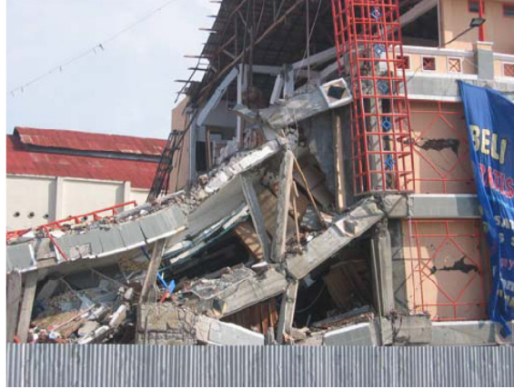
Fig. 1 Joint failures causing partial to total collapse of structures
