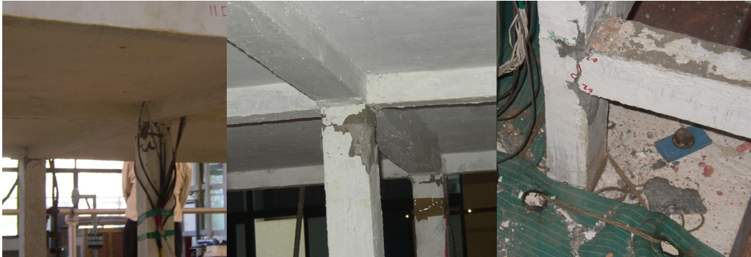
Fig. 19 Damage patterns observed at PGA = 0.5 g
