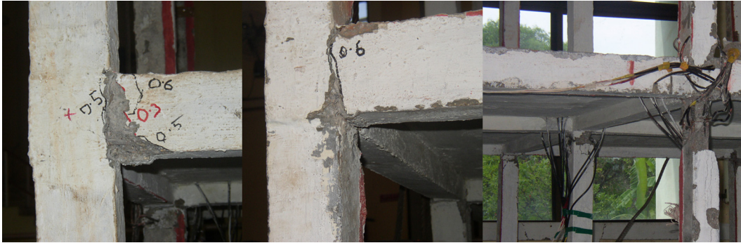
Fig. 20 Damage patterns observed at PGA = 0.6 g
